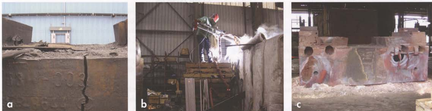
Figure 2. The operational sequence for the repair of a severely cracked forging hammer base: a) the fractured base before repair; b) workman repairs hammer base using Weld Mold's welding arm apparatus; and c) the finished repair.
